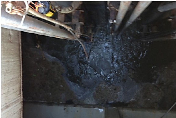
Without Air Blower Slight Grease Cap in Corners
