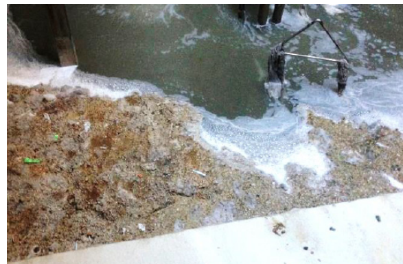
Breaking the Floating Grease Cap
