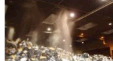
BOC ODOR CONTROL USING MISTING SYSTEM
