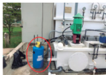
FIGURE 3. BOC storage and dosing tank.
