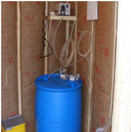
Electrical/Pump Set up
