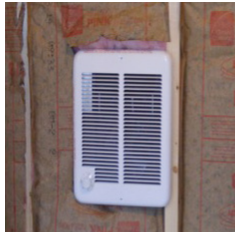
Storage Shed Heater
