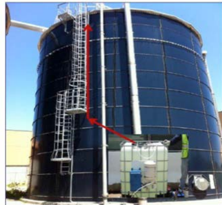
BOC Misting System Installed Into 12" Exhaust Vent and Tote Bin Location
