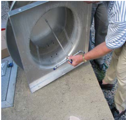
ESP Misting System Installed In 12" Vent
