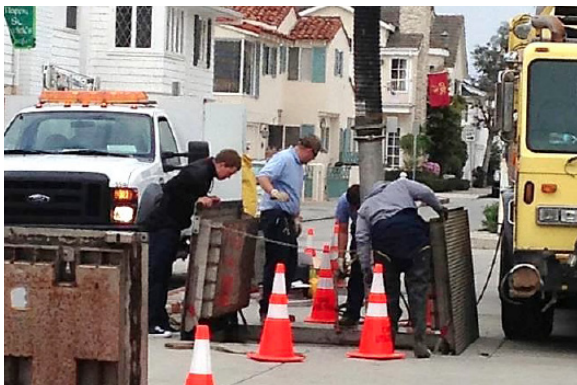
Vacuum Cleaning of Pump Station
