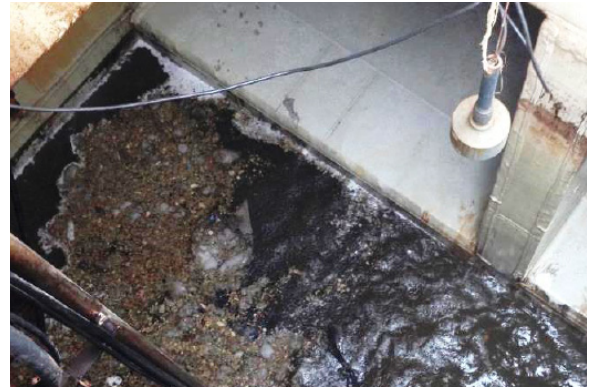
Highly Degraded Floating Grease Cap
