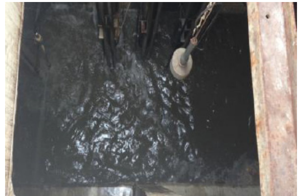
With Air Blower No Grease Caps Remaining
