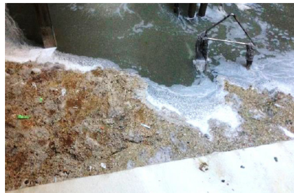
Breaking the Floating Grease Cap
