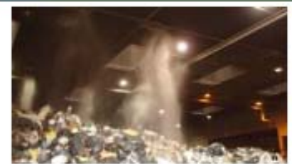
BOC ODOR CONTROL USING MISTING SYSTEM
