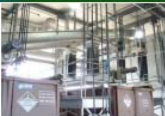
Mississauga WWTP, Canada-Odor Control For the Grit Screening Screw Conveyor Operation
